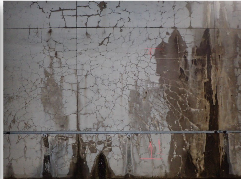
West retaining wall cracking & seepage
