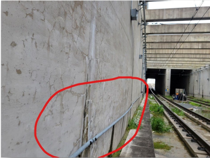
Bulging area in the west retaining wall
