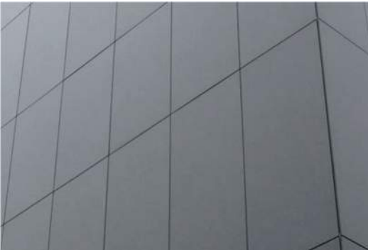
WALL FINISH 04 HORIZONTAL CONNECTOR PASSIVE WALL Material: GFRC cladding Color: Natural concrete color Size: TBD Surface Finish: Smooth BOD Product: FibreC Alternate: Architectural cast-in-place concrete
