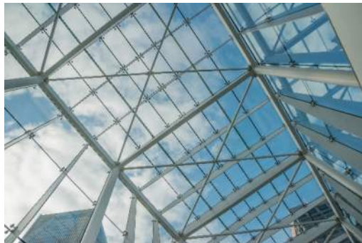
Entrance shaft natural lighting– MBTA Government Center Station
