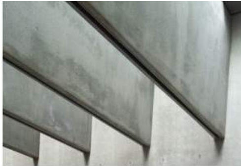
CEILING FINISH 01 ENTRY PAVILION CEILING (MAIN & SECONDARY) Material: Exposed architectural concrete structure Color: White Surface Finish: Smooth BOD: BPD white precast Alternate: Molded GFRC over steel structure
