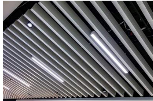
CEILING FINISH 02 HORIZONTAL CONECTOR CEILING Material: Suspended acoustic metal baffle ceiling Color: Grey Surface Finish: Smooth, perforated BOD Product: Linder baffle ceiling, Certainteed Tavola
